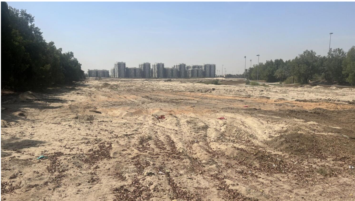
Ground has been broken on the redesign of the Garden Course at Abu Dhabi Golf Club
